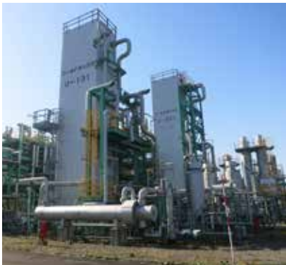
Air Products' LNG cold boxes installed at a plant site in Hokkaido, Japan (courtesy of JAPEX).
