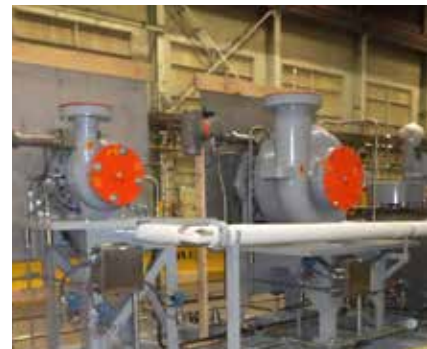
Air Products' cryogenic expander installed in a small-scale LNG plant.
